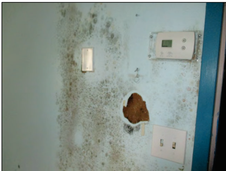
TYPICAL INTERIOR VIEW OF MOLD IN MAIN HOSPITAL FACILITY
