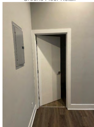
In unit Electric Panel
