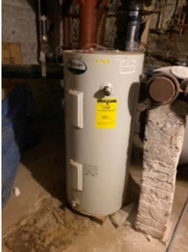
Hot Water Heater
