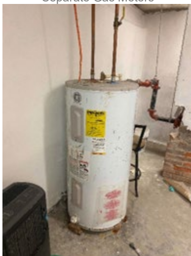
Hot Water Heater
