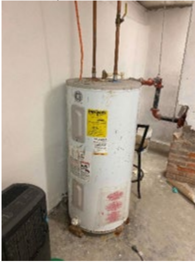
Hot Water Heater
