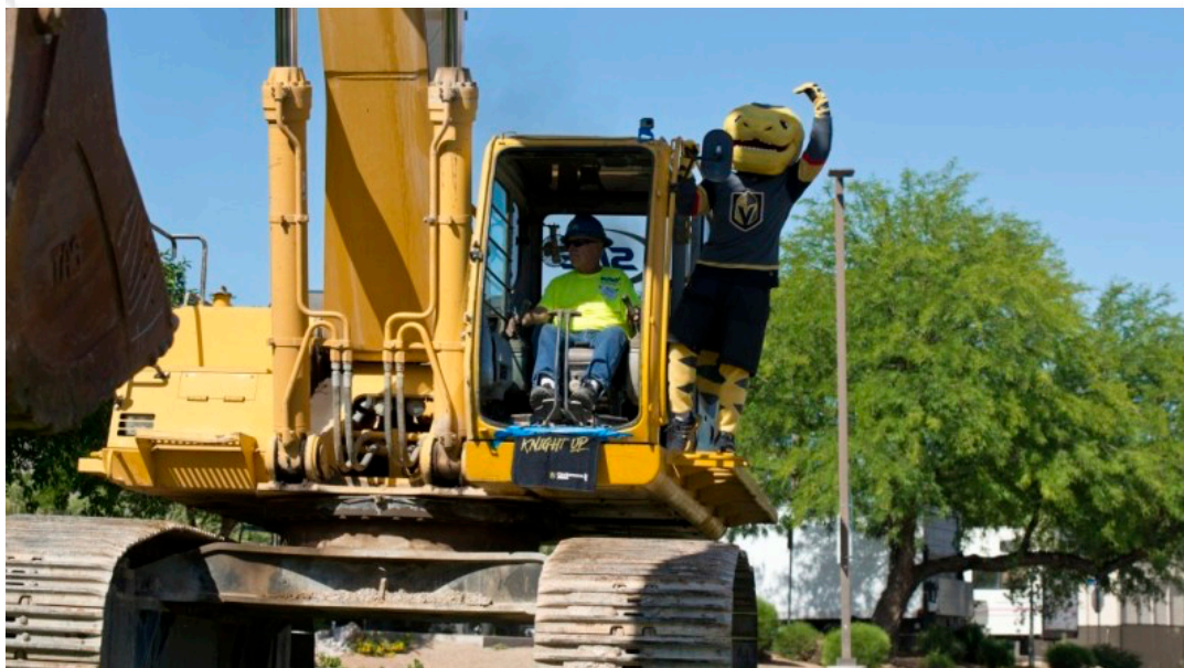
The Golden Knights' mascot, Chance, participates in a demolition event to start the ice center center project in Henderson.
